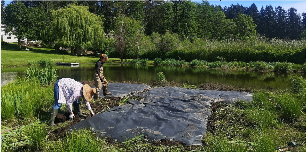
Elodie Roger (SMWS Staff) and Stephanie Cottell (CVLT) install sheets of pond liner over invasive Yellow Flag Iris on Somenos Lake
