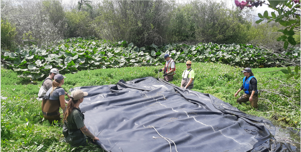
SMWS Staff and MNC Staff install the first sheets of pond liner over Parrot's Feather on Somenos Creek
