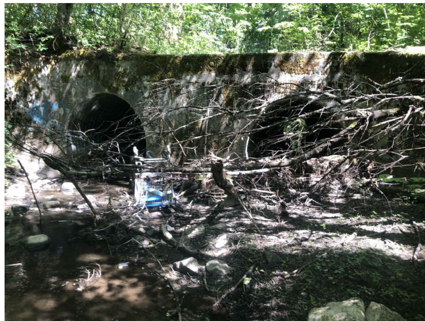
R3 – Double culvert at foot trail with debris and garbage
