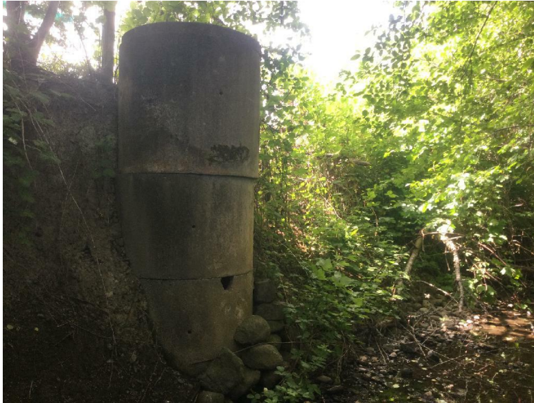
R3 – Old farm well now in creek due to erosion.
