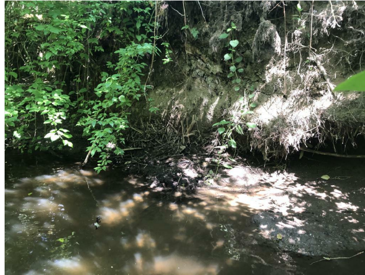
2.) Placemark 6- Reach 2, Pool 2. Heavy erosion along left bank
