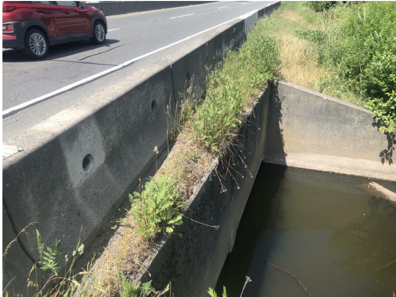
3.) Placemark 28- Reach 1, highway culvert barely above summer water level
