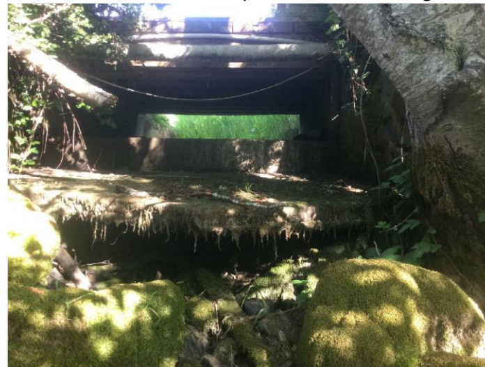
R3 – Golf course spill way is eroding (Duncan Meadows)
