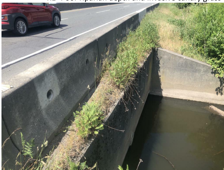
R1- Highway runoff goes straight to creek
