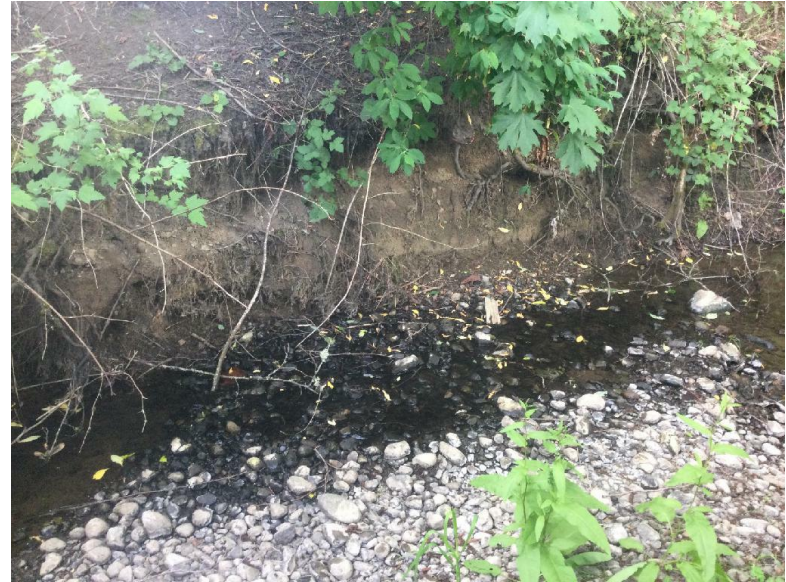
R3 – Heavy bank erosion on river right.
