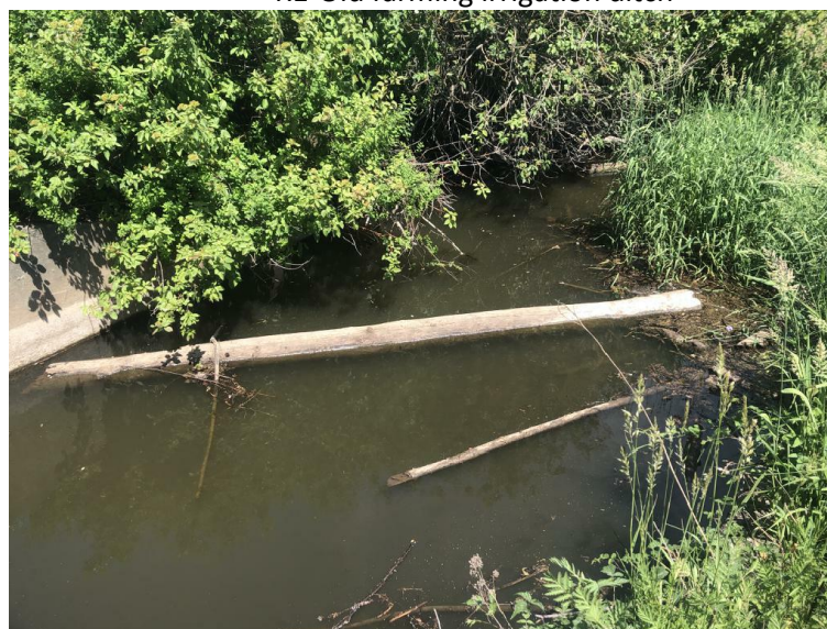
R1- Highway sump needs to be dredged
