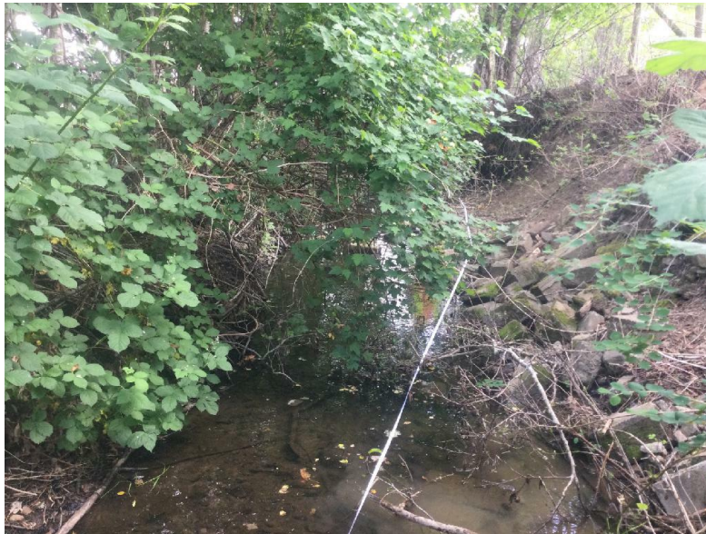
R3 – Old concrete falling into the creek
