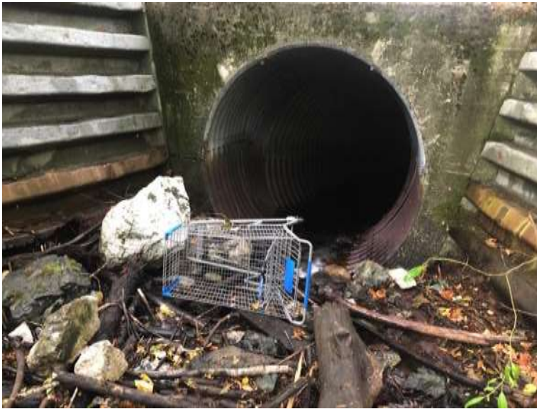
R5 – Garbage and debris plugging CV Culvert (Site 50)
