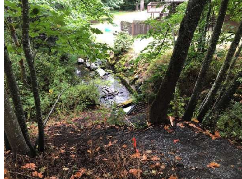
4.) R4 ends at CV Trail barrier culvert, Veg removal on right bank
