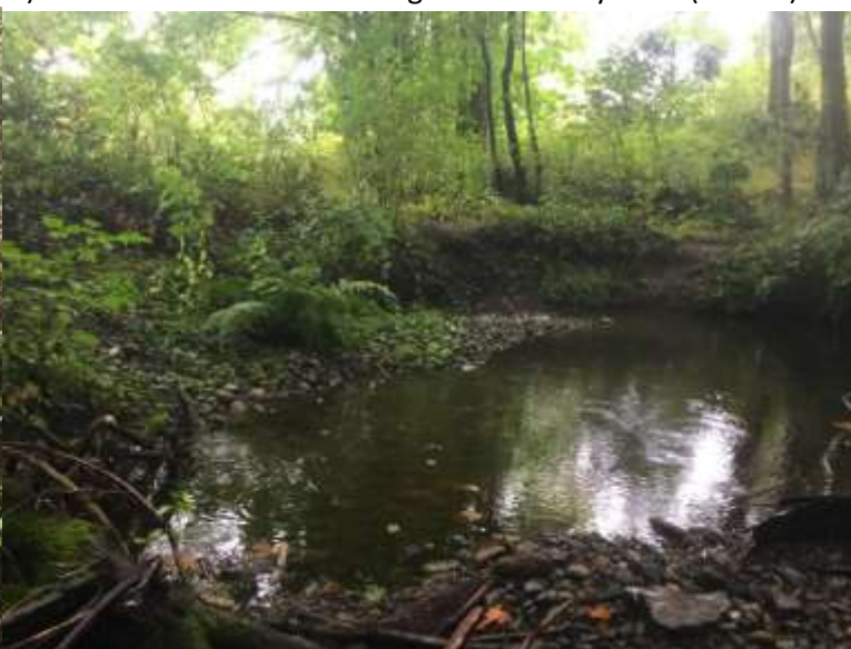
R6 – CV Trail Culverts opposite bank erosion.
