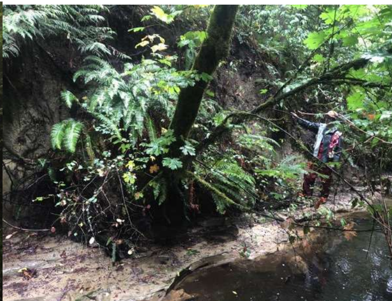
R6– Eroding left bank Clay bank (Site 92).
