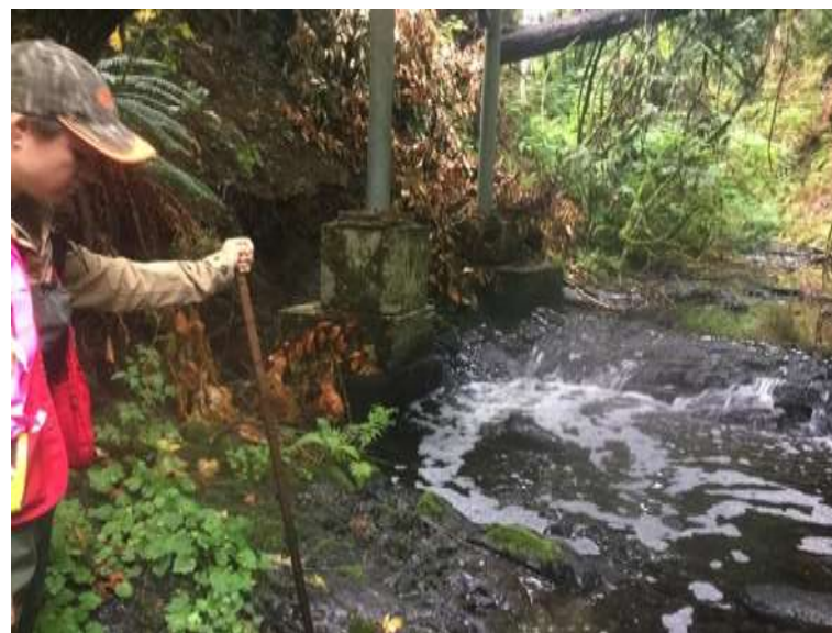
R4 - Driveway Bridge footing erosion. (Site 43)
