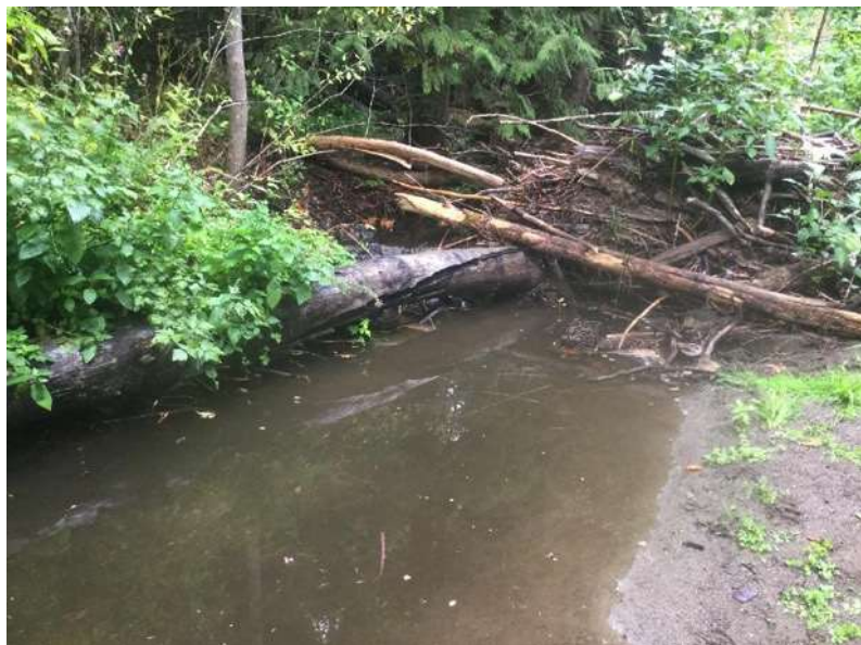
R3 -Log jam has garbage deposits as well, needs cleaned.
