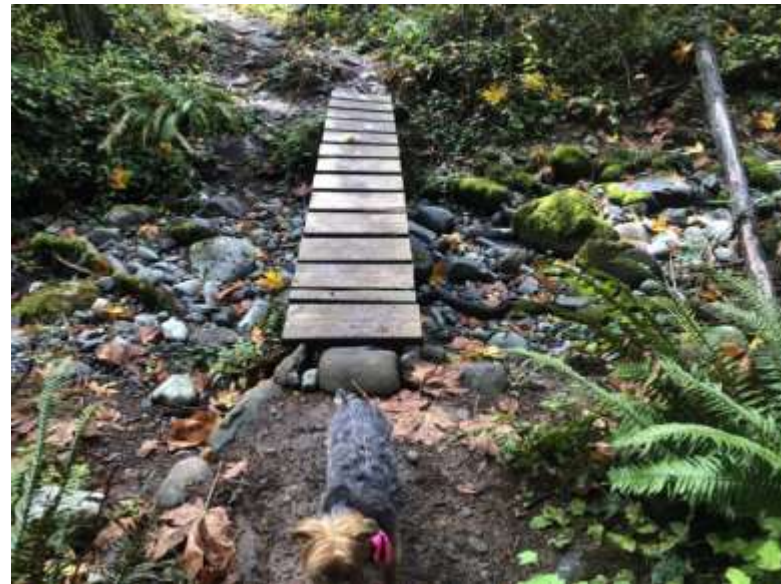
2.) R8- Footbridge is inadequate size, results in stream walking
