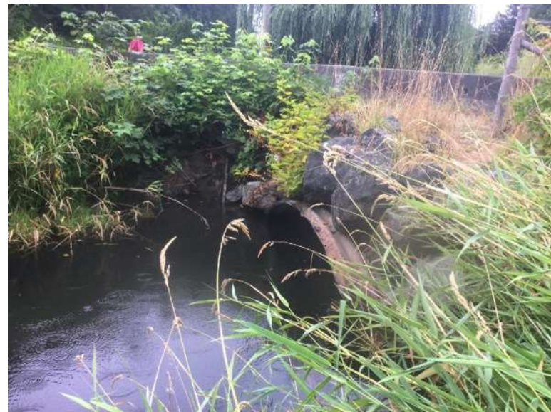
R2 Beaver flooding Mary St culvert
