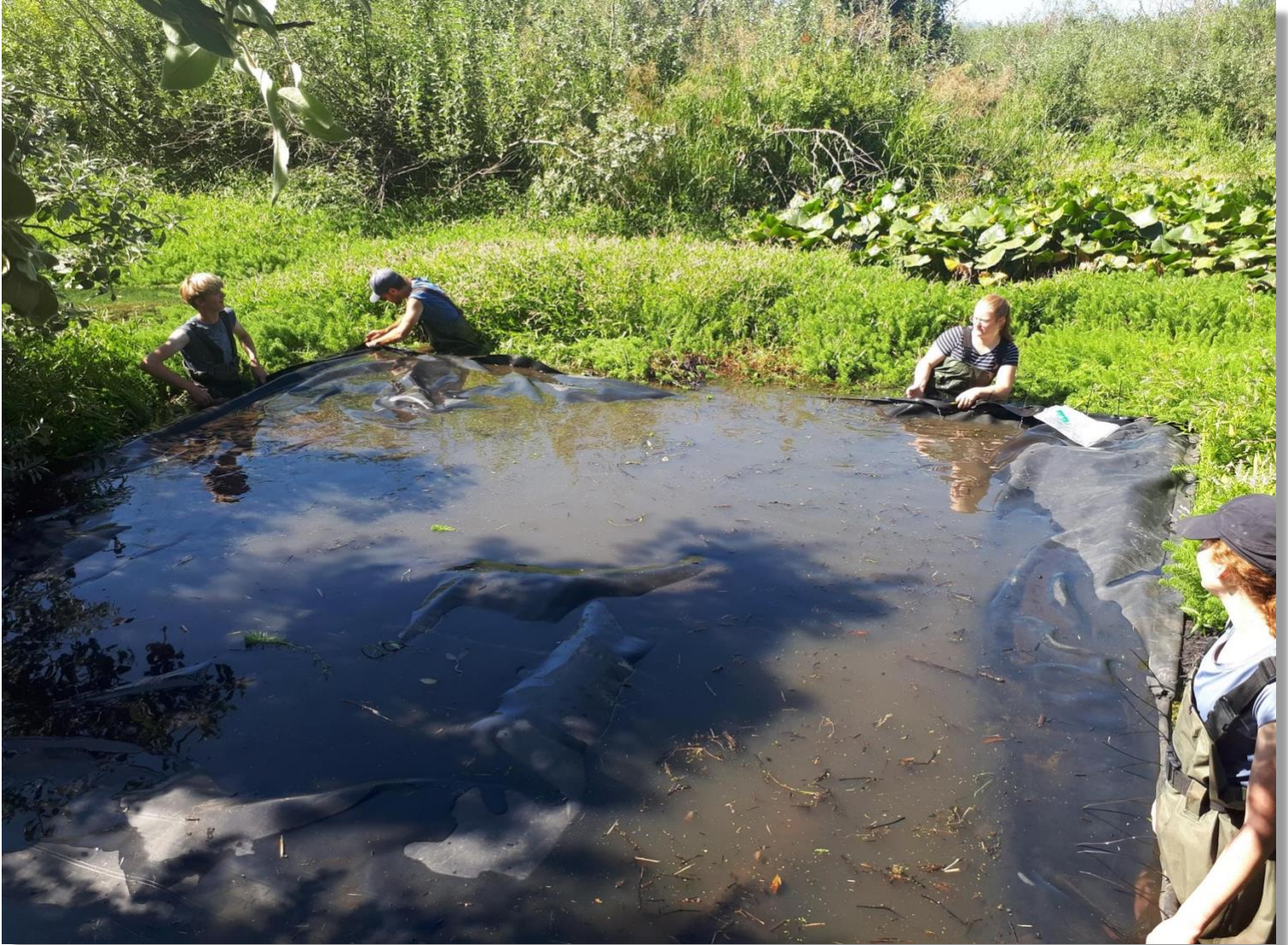
Photo: SMWS staff members install a sheet of pond-liner to be used as test treatment for the parrot's feather invasion. Photo By: Amanda McKinnon
