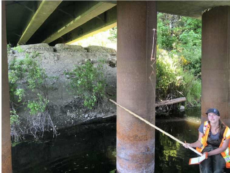
R1A- Herd Rd Bridge erosion.
