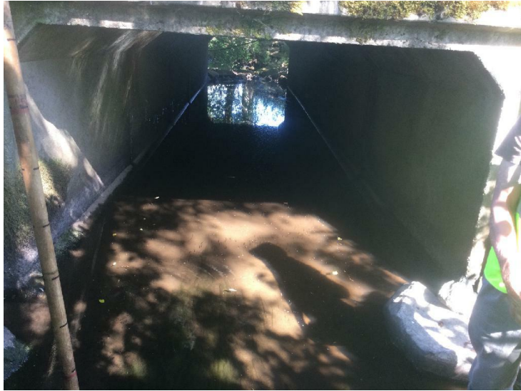
1.) Reach 2, Pool 1- Richards Trail box culvert full of coho fry.
