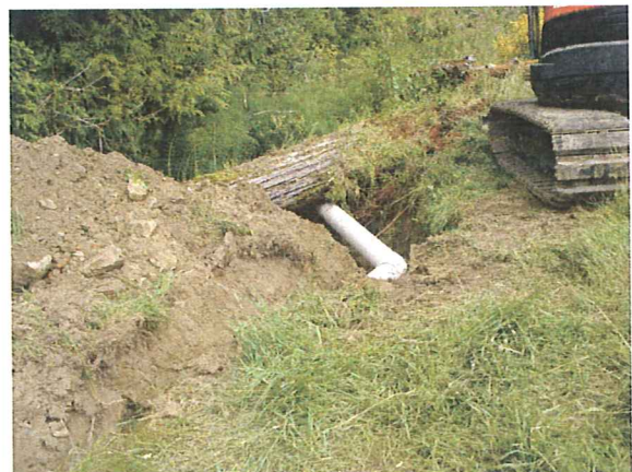
Photos 4 and 5. New, larger diameter pipe laid below Crofton Lake dam, to enable an increased release rate to Richards Creek. Upgrades occurred in June 2008, overseen by District of North Cowichan engineering staff.
