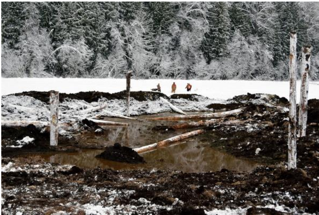
This emergent wetland was built in less than one day at Meadow Creek. Note how the soil was piled to provide planting sites for trees and shrubs. Logs were placed in the wetland for woody debris, and set for snags
